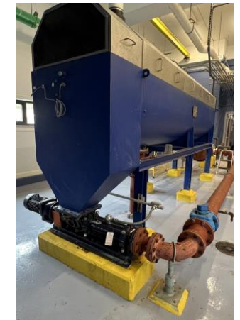
Figure 3 - WAS Thickener and Thickened Sludge Pump
